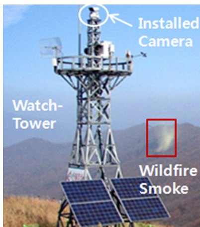
Fig. 2 CCD camera mounted on a watchtower for wildfire detection, taken from Ref. 11.
